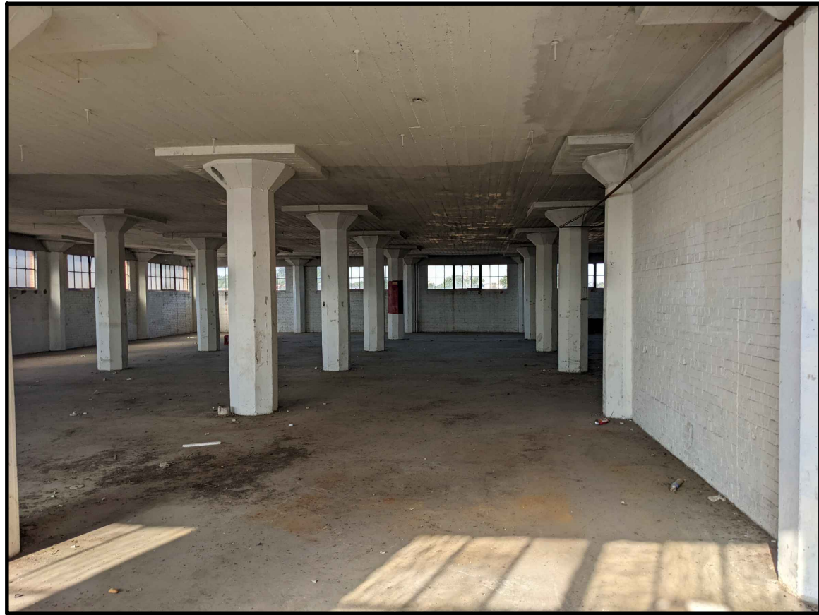
2ND FLOOR – EXISTING PHOTO EXISTING BRICK WALLS – PAINTED: REPAIR, REPLACE AND TUCKPOINT DAMAGED AREAS. REMOVE LOOSE PAINT AND DEBRIS. CLEAN AND PREP FOR NEW PAINT. EXISTING PAINTED COLUMNS, COLUMN CAPS AND CEILING DECK. REMOVE LOOSE PAINT AND DEBRIS. REPAIR DAMAGED AREAS. PREP FOR NEW PAINT.
