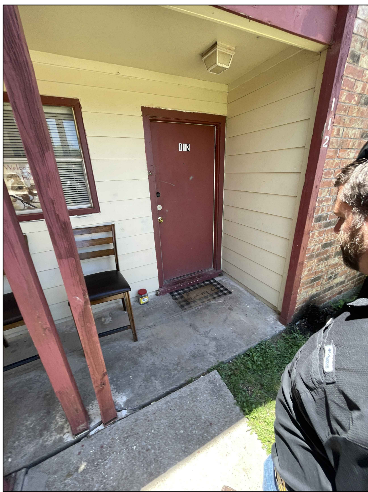
EXISTING CONDITIONS. EXISTING CONCRETE WALK/SLAB AT NEW ACCESSIBLE UNITS WILL NEED CORRECTION TO ELIMINATE "STEP". REF. CIVIL
